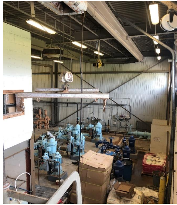
Plant Room – High and Low Lift Pumps
