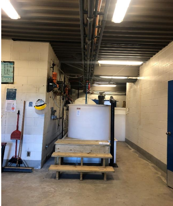
Main floor - chemical feed room
