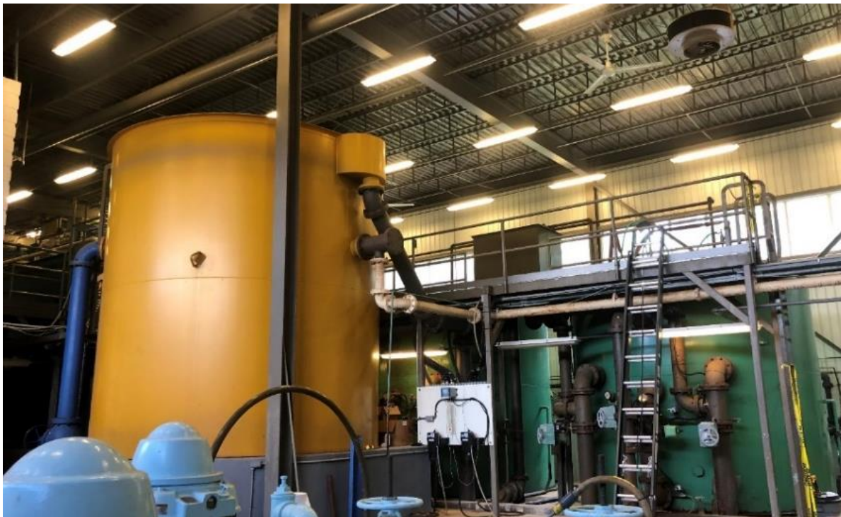
Plant Room – Pre Contact Tank and Clarifiers
