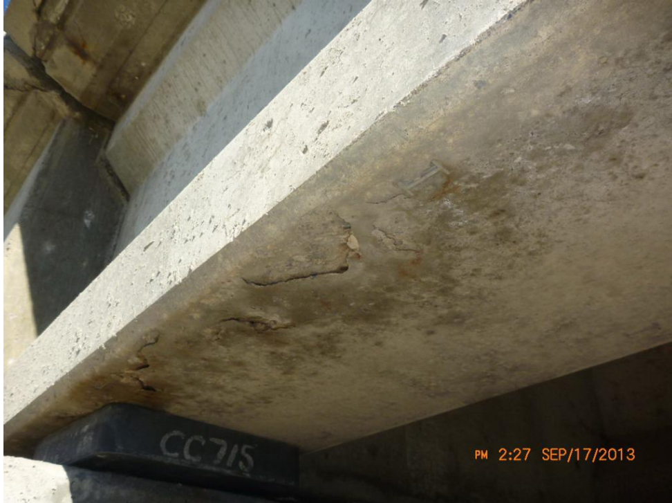
Comments: DELAMINATION AT GIRDER END
