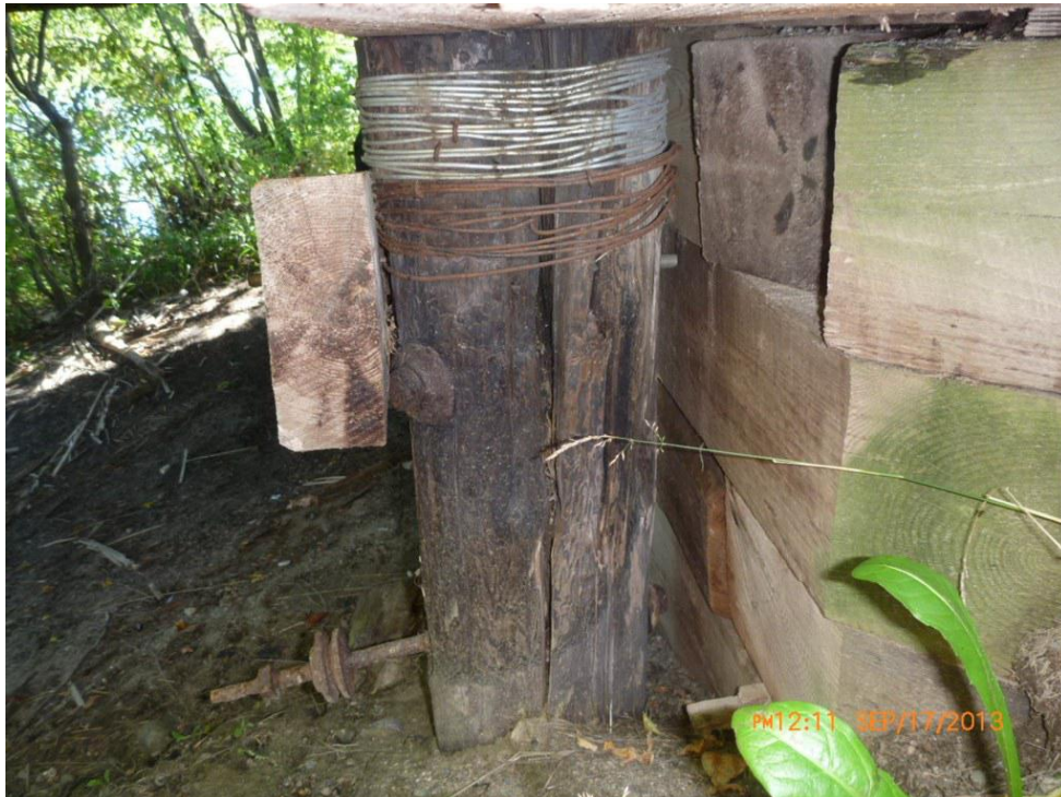
Comments: SEVERE SPLITTING OF ABUTMENT PILE
