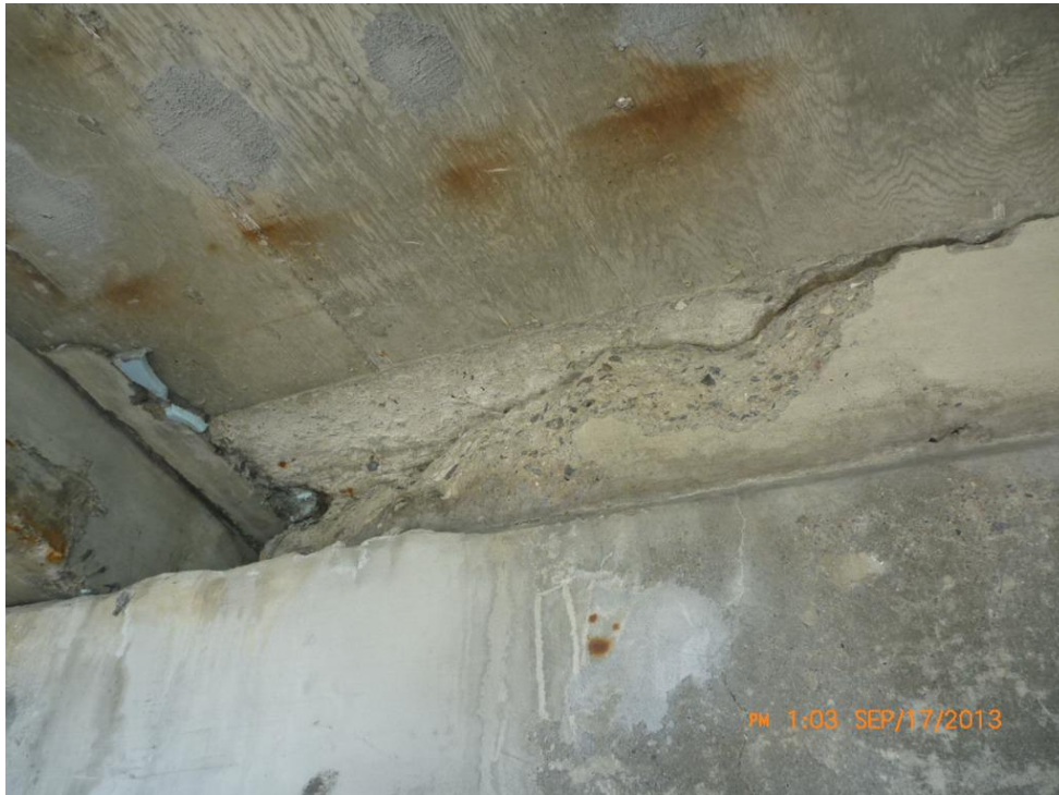
Comments: SPALLING OF ABUTMENT DIAPHRAGM
