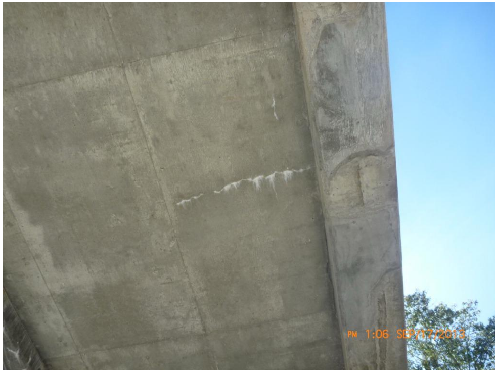
Comments: NARROW STAINED CRACK ON DECK SOFFIT
