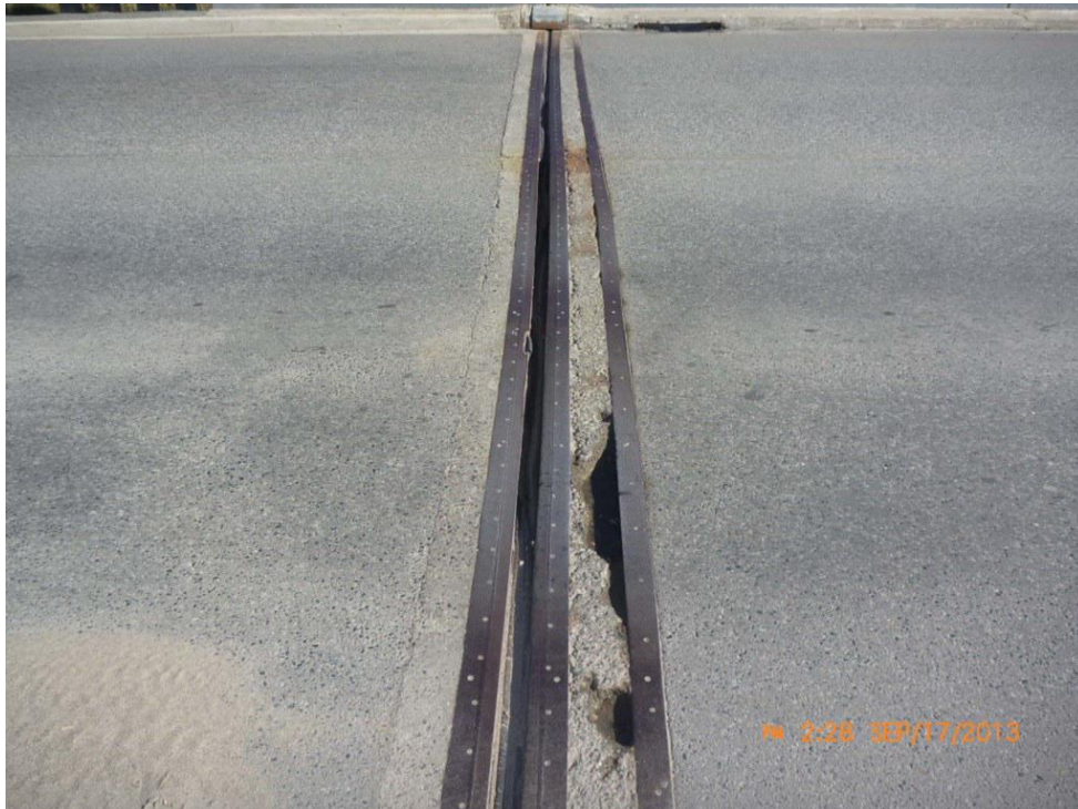
Comments: EAST EXPANSION JOINT
