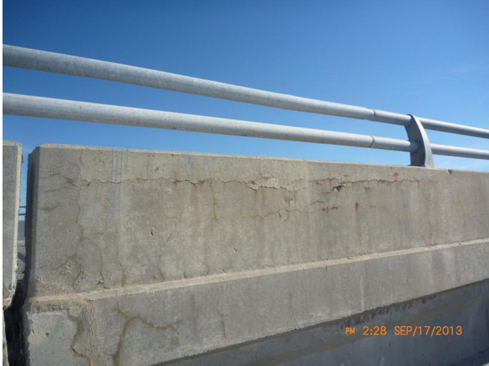
Comments: DELAMINATION ON BARRIER WALL
