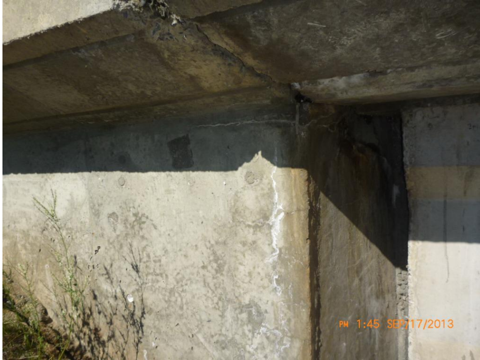
Comments: EFFLORESCENCE ON WINGWALL
