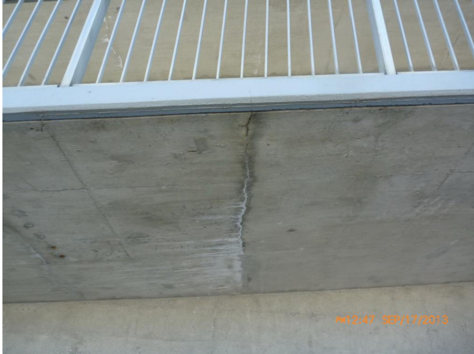
Comments: NARROW STAINED CRACK ON PEDESTRIAN WALKWAY SOFFIT
