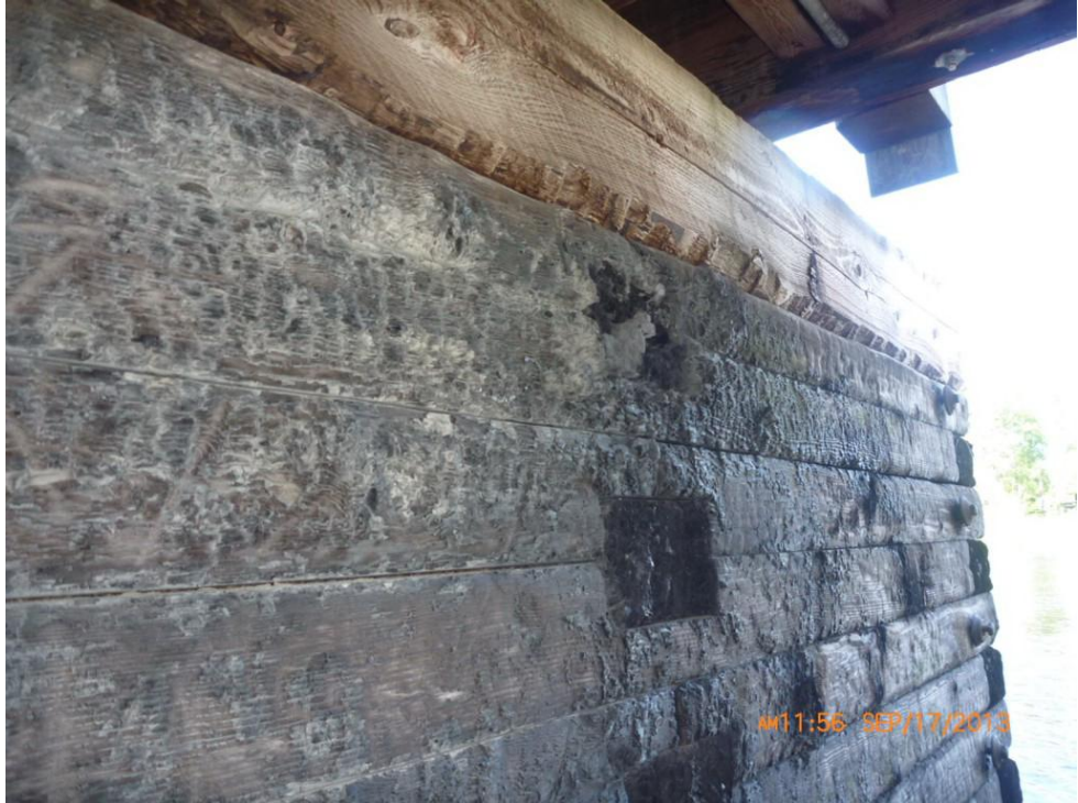
Comments: FIRE DAMAGE ON EAST PIER SHEETING
