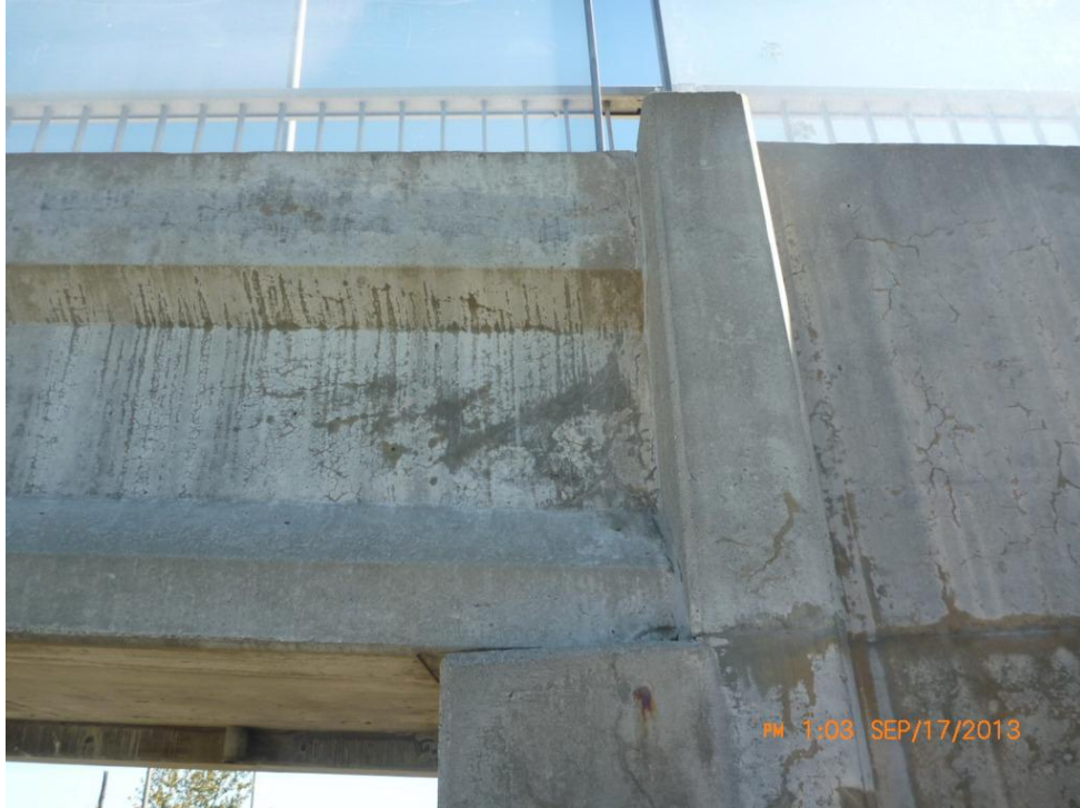
Comments: DIAGONAL CRACKING ON GIRDER END AT WEST ABUTMENT
