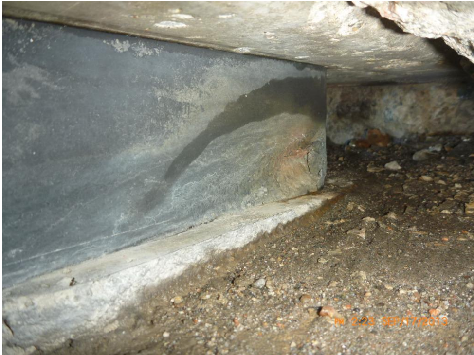
Comments: GOUGE OUT OF ABUTMENT BEARING PAD
