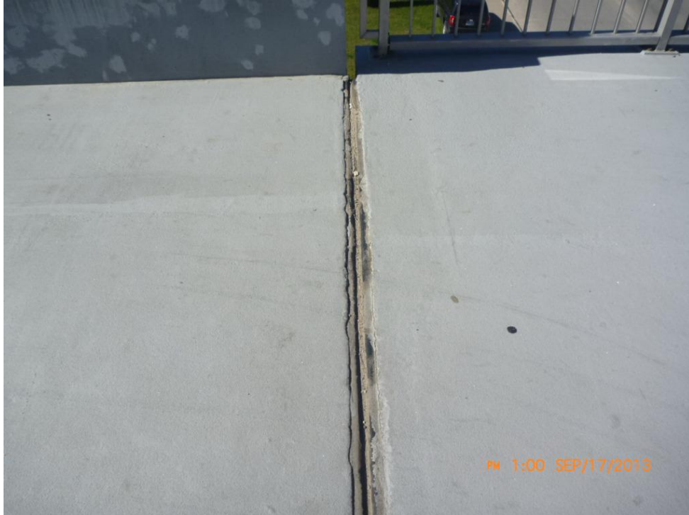
Comments: EAST EXPANSION JOINT
