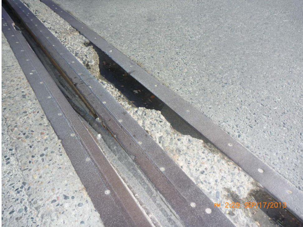
Comments: SEVERE SPALLING OF EAST JOINT END DAM
