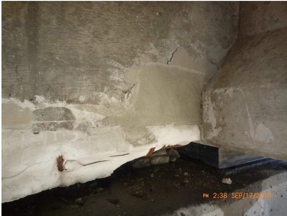
Comments: DEBONDED PATCH AT WEST ABUTMENT DIAPHRAGM
