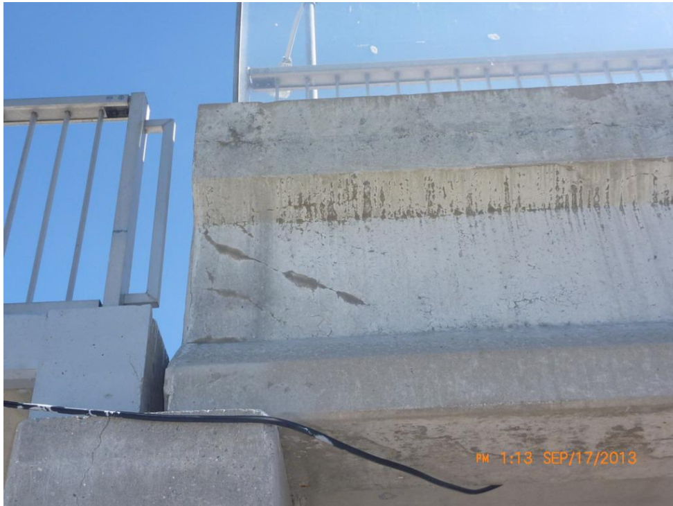
Comments: DIAGONAL CRACKING ON GIRDER END AT EAST ABUTMENT Path: E:\WorkTech Data\Chapleau\Photos\2013\Photo 049.JPG
