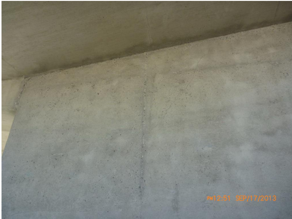
Comments: DIAGONAL CRACK ON ABUTMENT
