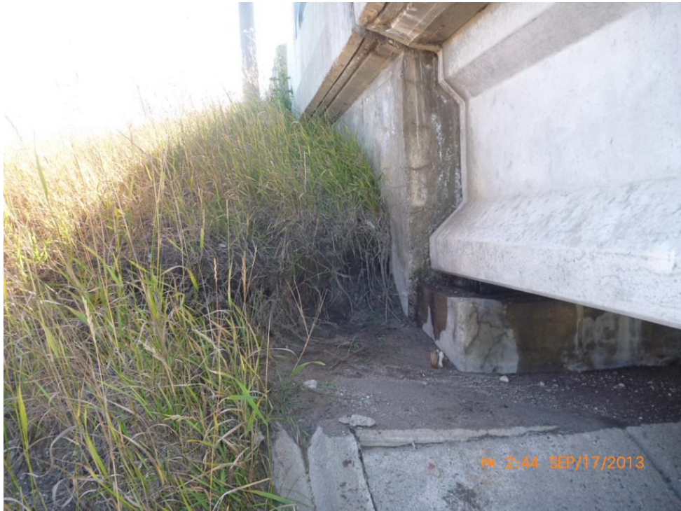
Comments: SEVERE EROSION OF EMBANKMENT
