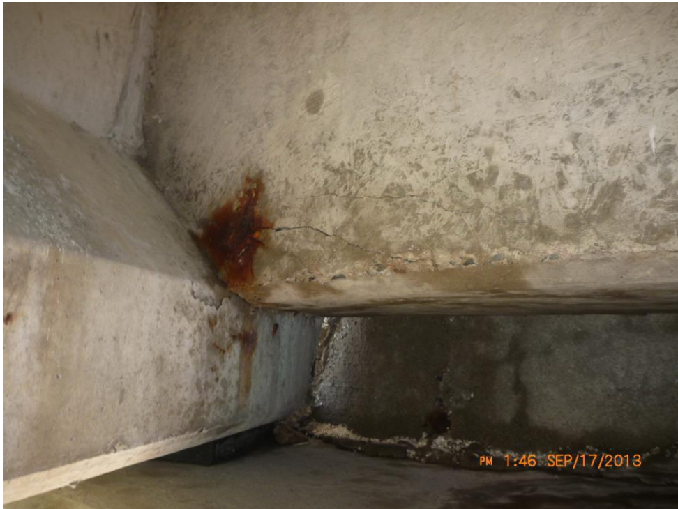
Comments: DELAMINATION ON DIAPHRAGM AT ABUTMENT
