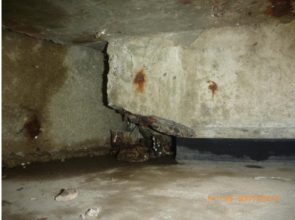
Comments: SPALL AND DELAMINATION ON GIRDER END
