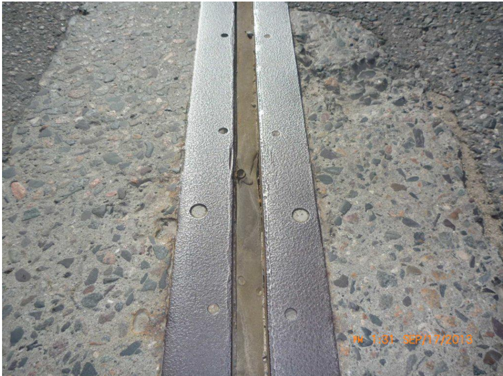
Comments: SEPARATION OF JOINT SEAL FROM ARMORING ANGLE Path: E:\WorkTech Data\Chapleau\Photos\2013\Photo 056.JPG
