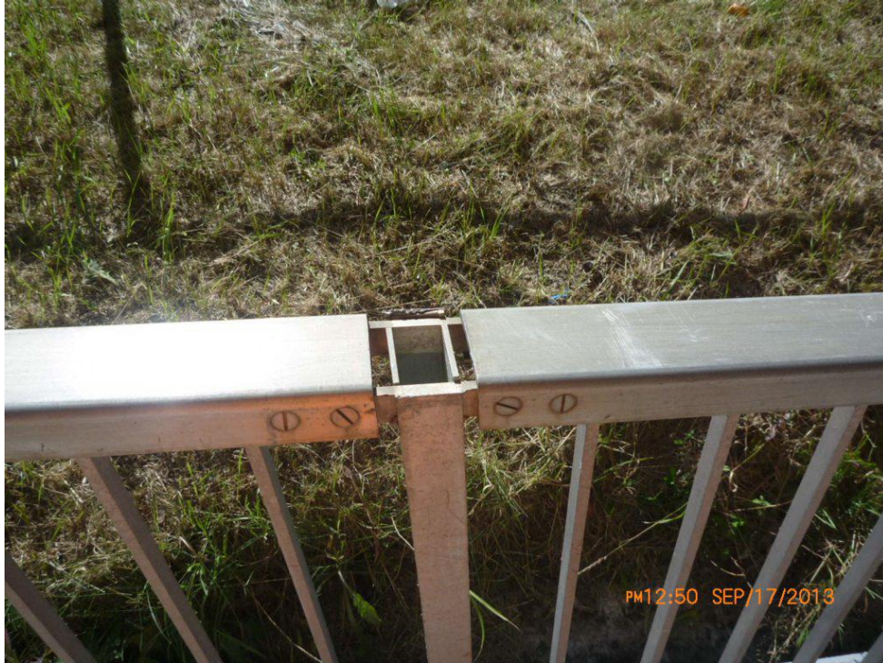
Comments: MISSING HANDRAIL CAP
