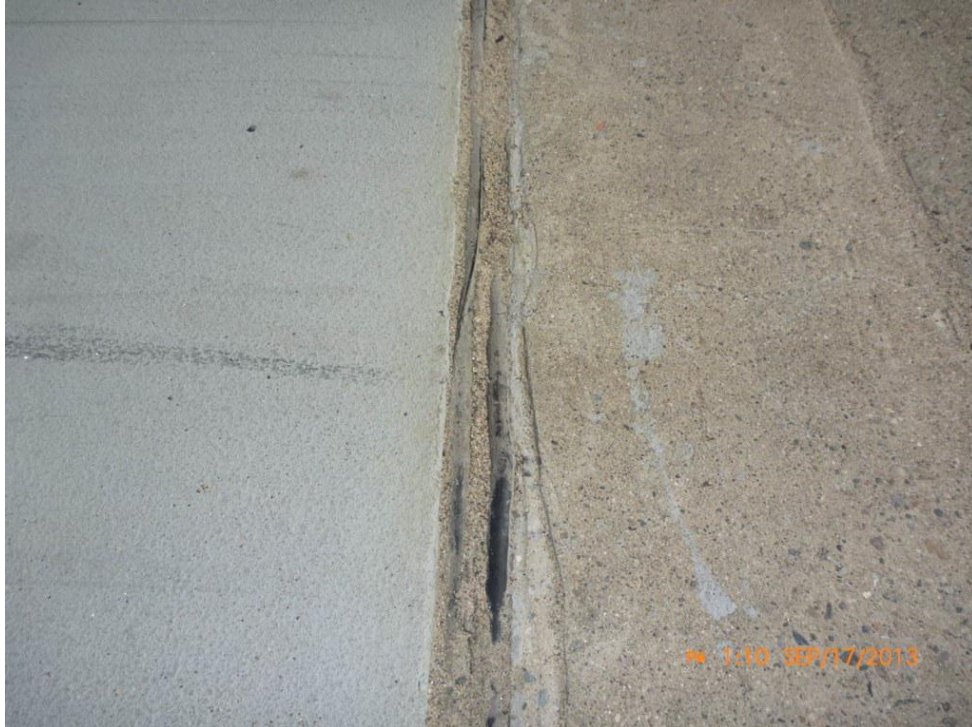
Comments: DEFORMATION OF WEST EXPANSION JOINT SEAL
