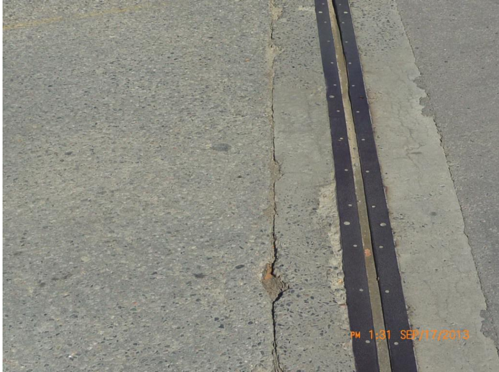
Comments: GAP BETWEEN APPROACH SURFACE AND JOINT Path: E:\WorkTech Data\Chapleau\Photos\2013\Photo 055.JPG
