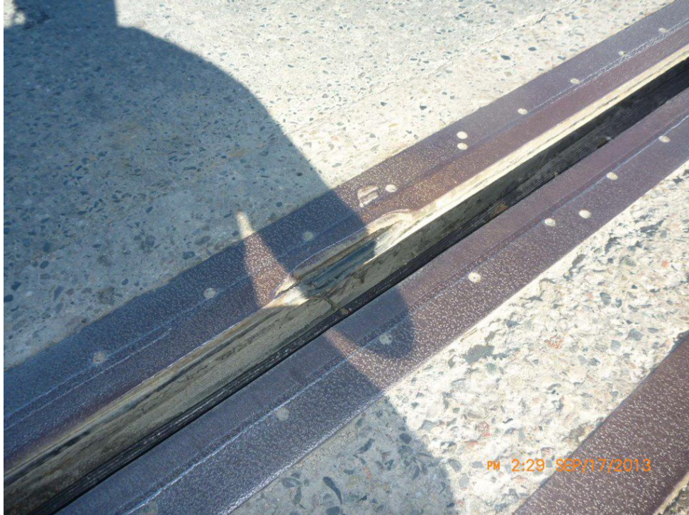
Comments: MISSING SECTION OF ARMORING ANGLE
