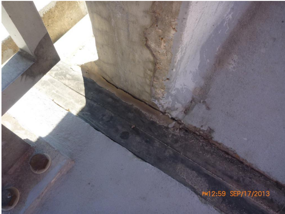
Comments: SEPARATION OF EAST SEAL FROM GIRDER
