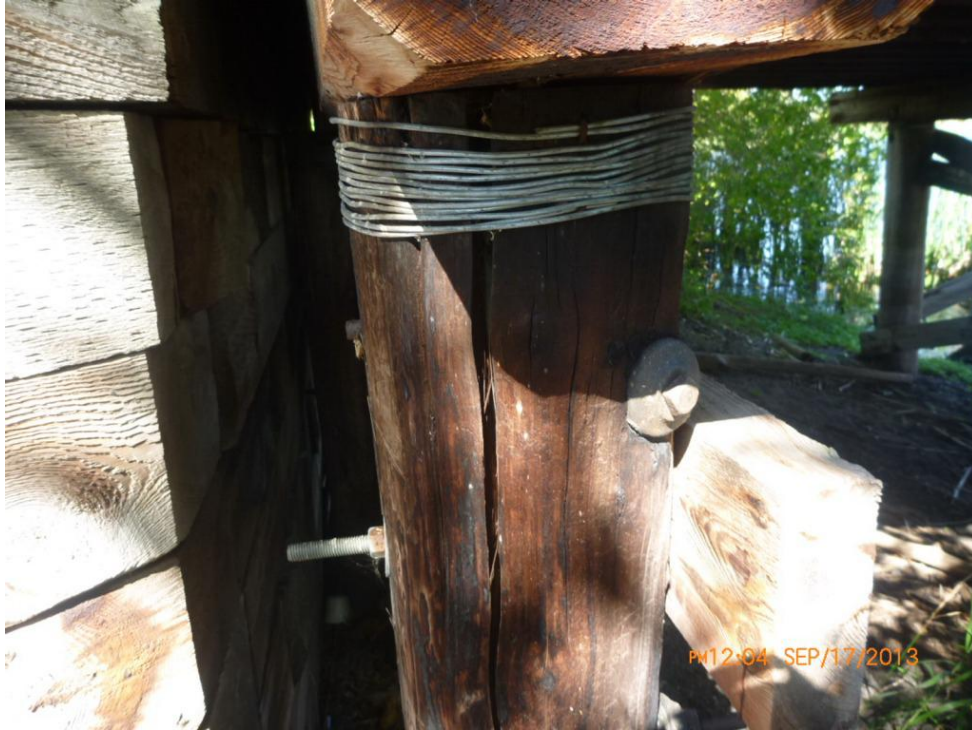
Comments: SEVERE SPLITTING OF WEST ABUTMENT PILE Path: E:\WorkTech Data\Chapleau\Photos\2013\Photo 014.JPG
