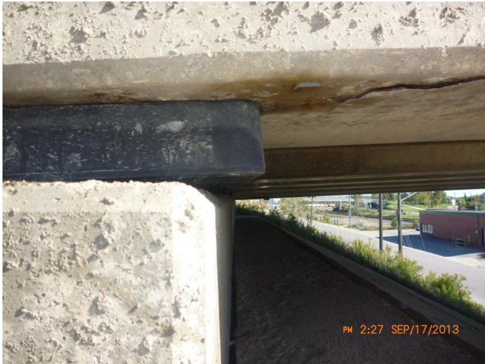
Comments: MOVEMENT OF BEARING PAD
