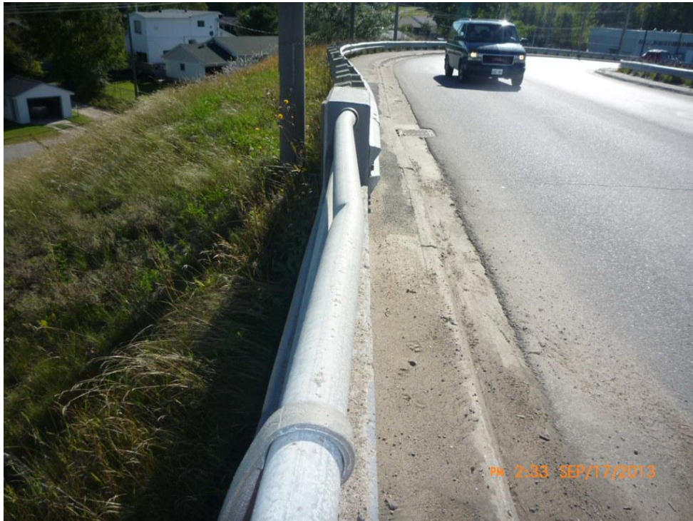
Comments: COLLISION DAMAGE TO HANDRAIL
