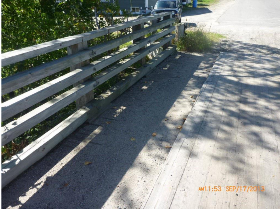
Comments: TYPICAL DECK TOP WITH DEBRIS
