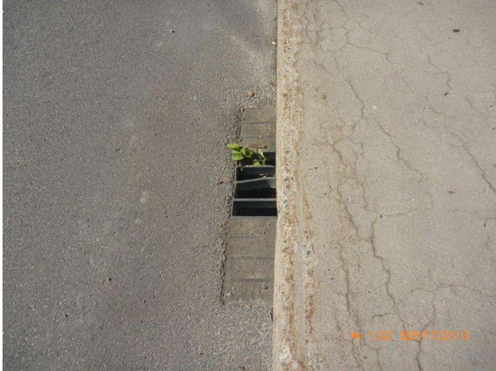
Comments: PARTIALLY PLUGGED DECK DRAIN
