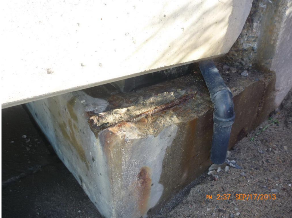
Comments: SPALLING OF ABUTMENT SEAT
