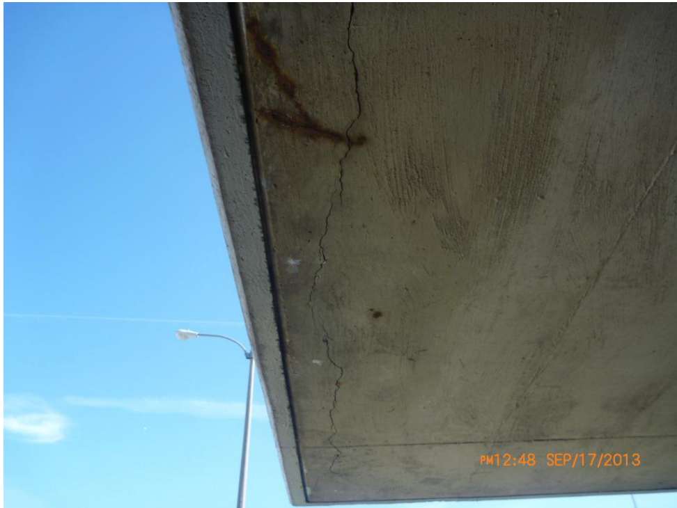
Comments: WIDE CRACK ON PEDESTRIAN WALKWAY SOFFIT
