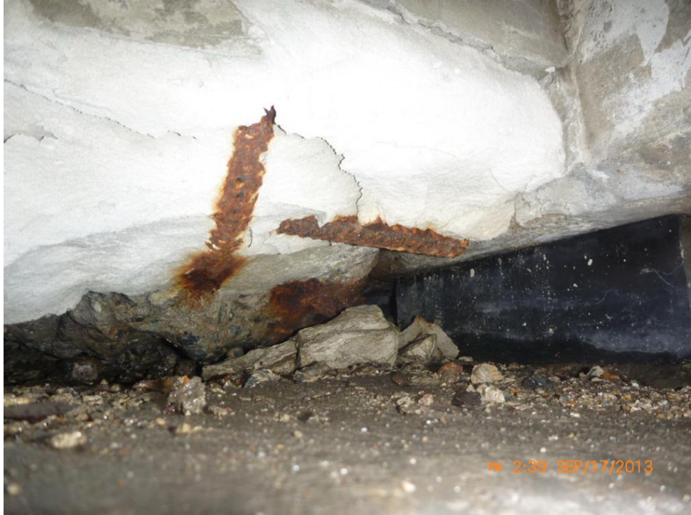
Comments: SPALLING OF WEST ABUTMENT DIAPHRAGM
