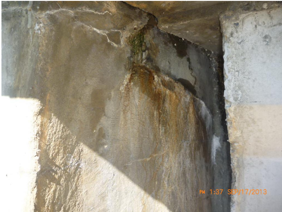
Comments: EFFLORESCENCE ON BALLAST WALL
