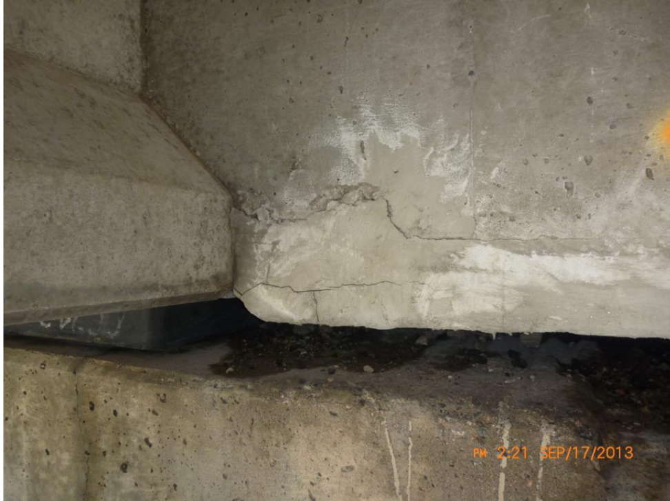
Comments: DEBONDED PATCH ON EAST ABUTMENT DIAPHRAGM
