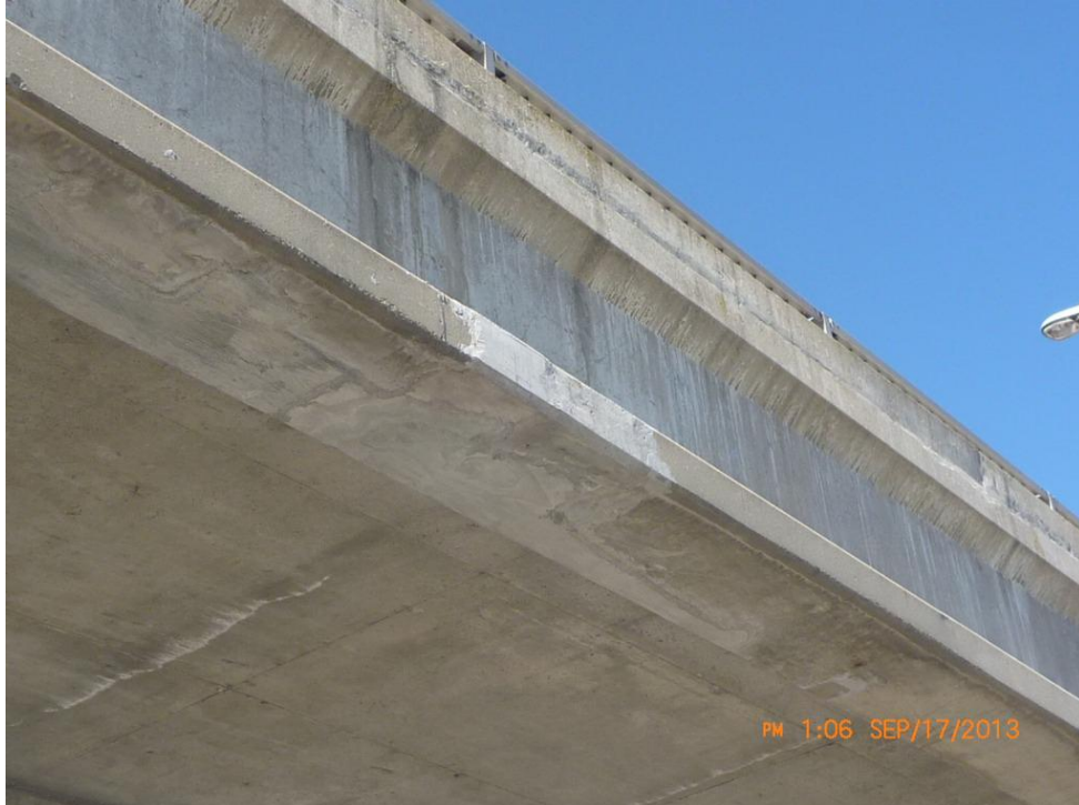
Comments: CONCRETE PATCH ON GIRDER
