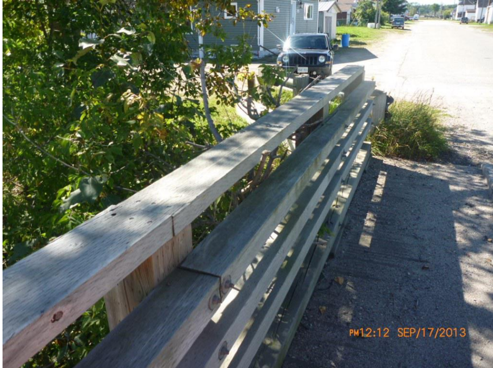
Comments: VEGETATION GROWTH THROUGH RAILING
