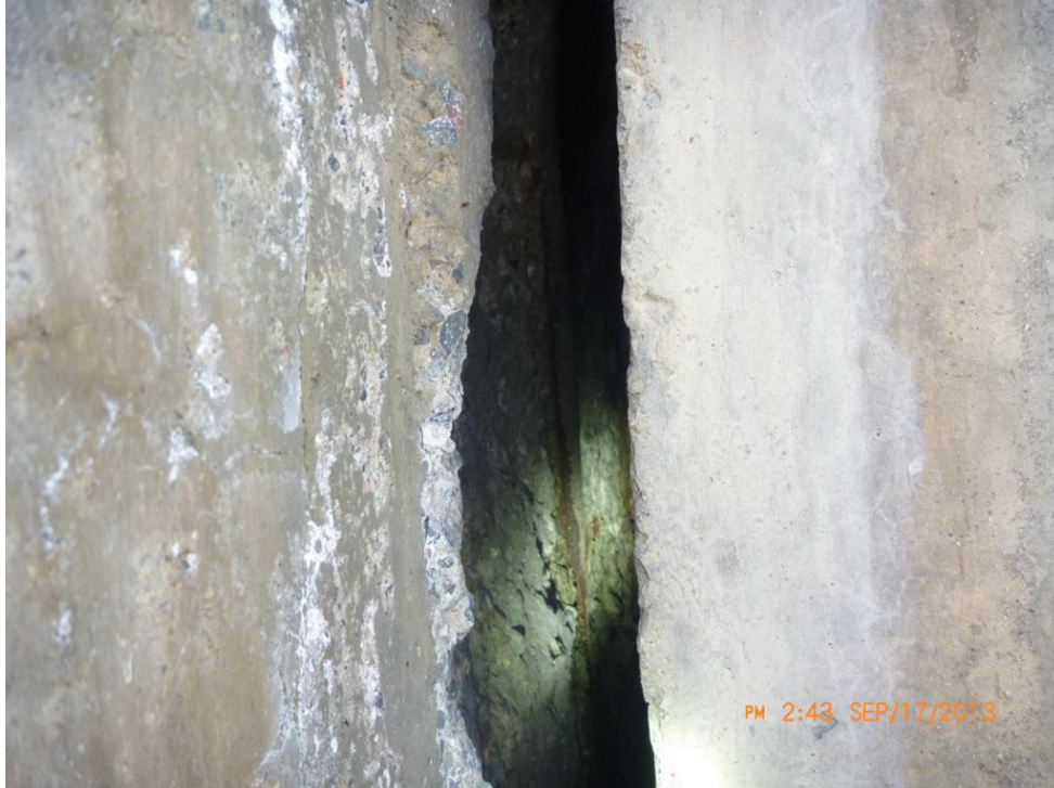
Comments: SEVERE SPALLING OF BALLAST WALL
