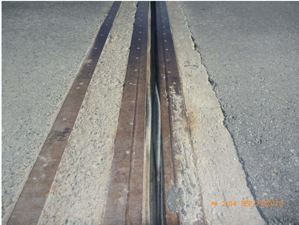
Comments: DEFORMATION OF WEST JOINT SEAL
