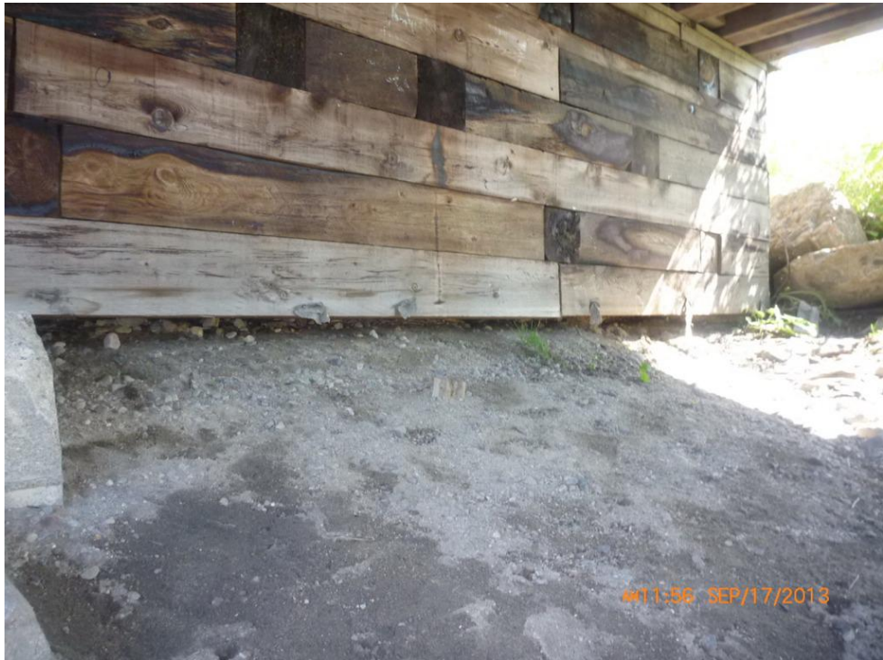
Comments: UNDERMINING OF EAST ABUTMENT WALL
