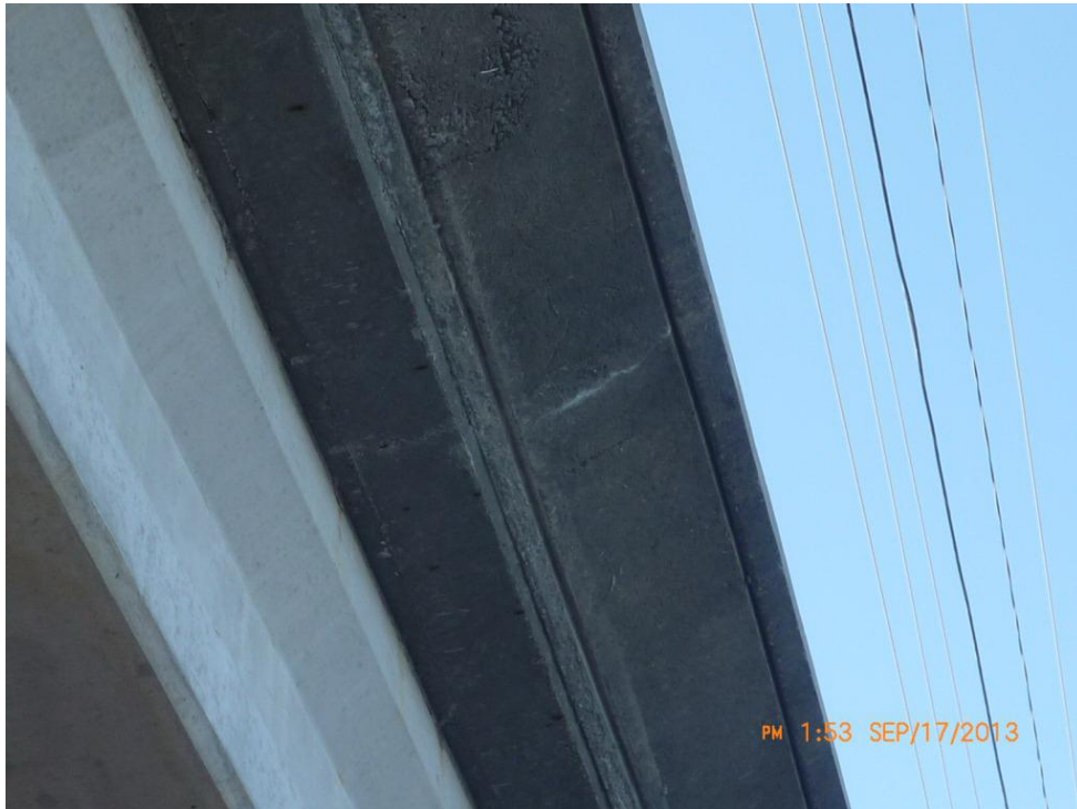
Comments: NARROW STAINED CRACK ON EXTERIOR SOFFIT
