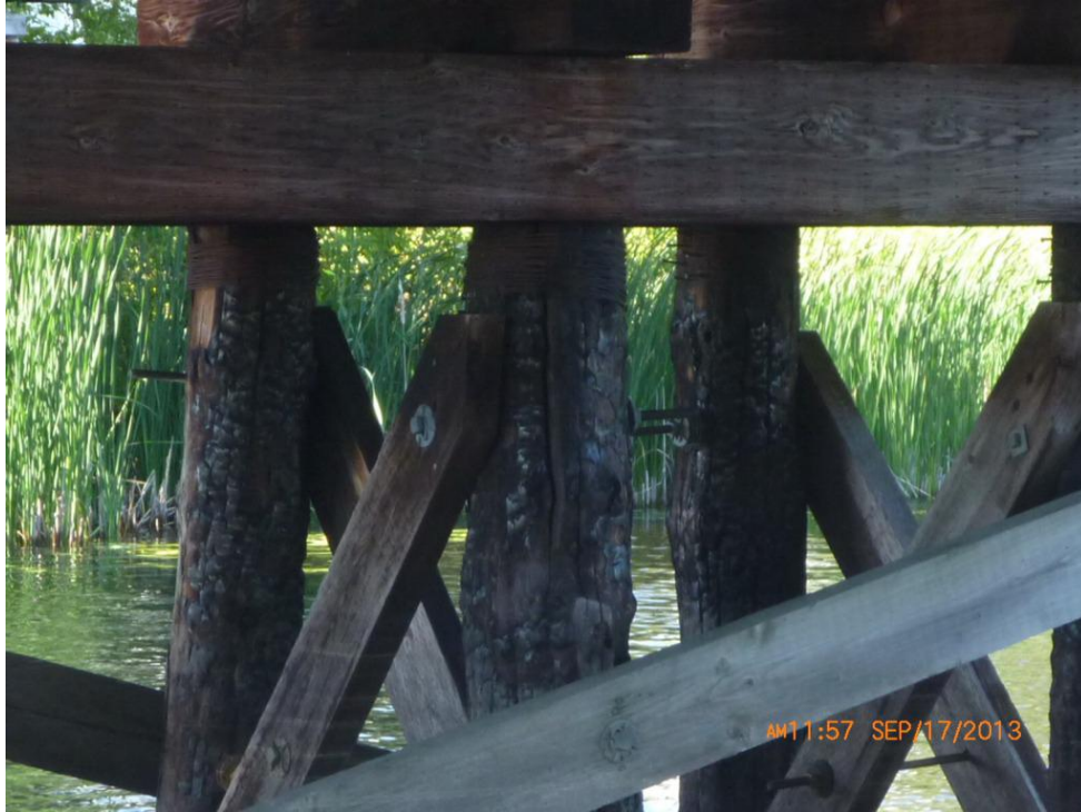
Comments: SEVERE SPLIT AND FIRE DAMAGE TO PIER PILE Path: E:\WorkTech Data\Chapleau\Photos\2013\Photo 012.JPG
