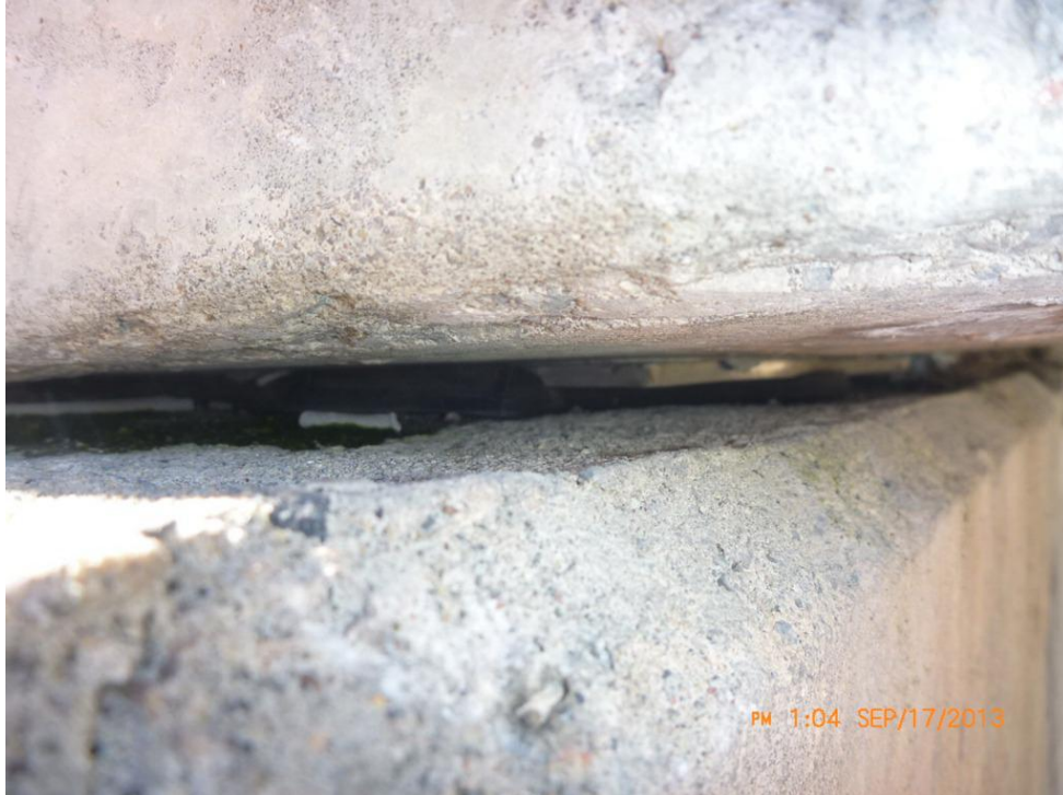
Comments: SQUASHING OF WEST ABUTMENT BEARING
