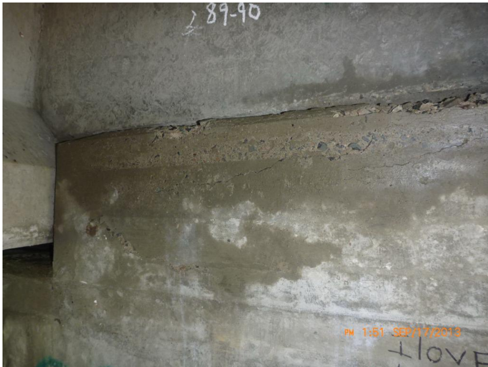
Comments: DELAMINATION ON ABUTMENT WALL
