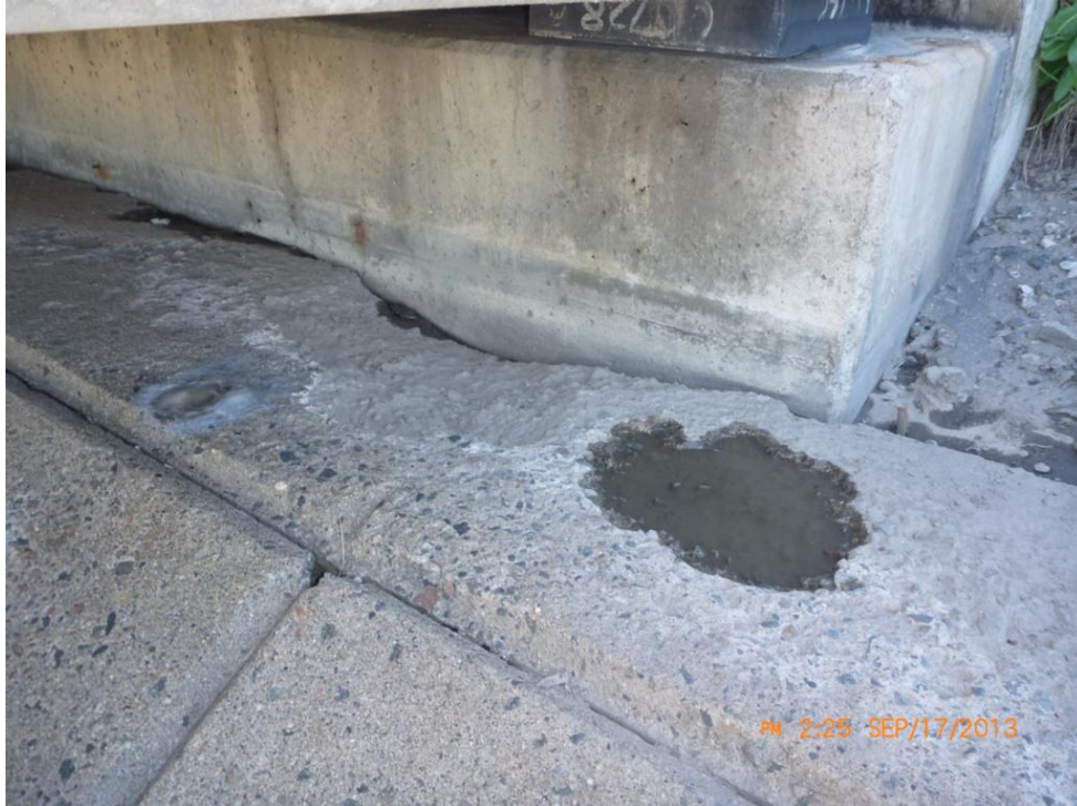
Comments: SEVERE SCALING OF SLOPE PROTECTION
