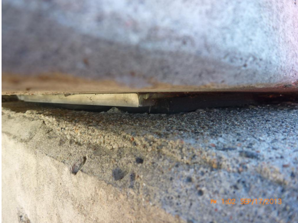
Comments: SQUASHING OF WEST ABUTMENT BEARING
