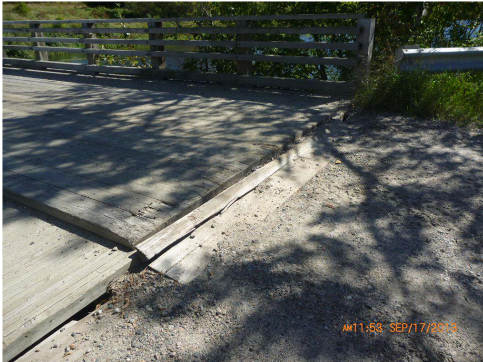
Comments: MISSING GRANULAR MATERIAL AT WEST APPROACH
