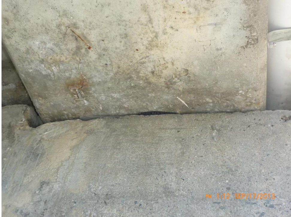
Comments: SQUASHING OF EAST ABUTMENT BEARING PAD Path: E:\WorkTech Data\Chapleau\Photos\2013\Photo 048.JPG
