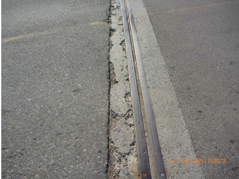
Comments: SEVERE SPALLING OF SOUTH JOINT END DAM
