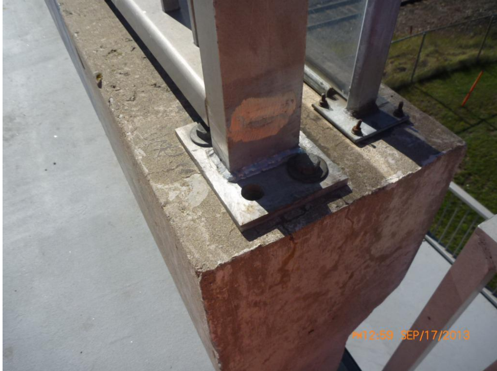
Comments: MISSING HANDRAIL BOLTS
