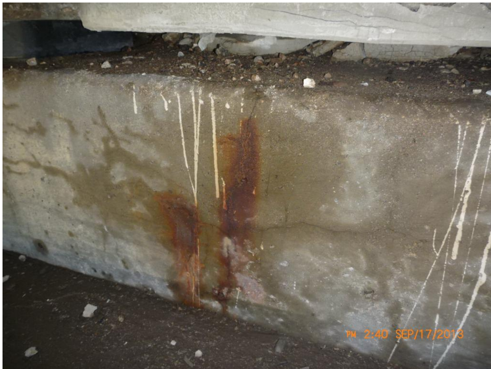
Comments: DELAMINATION ON ABUTMENT WALL
