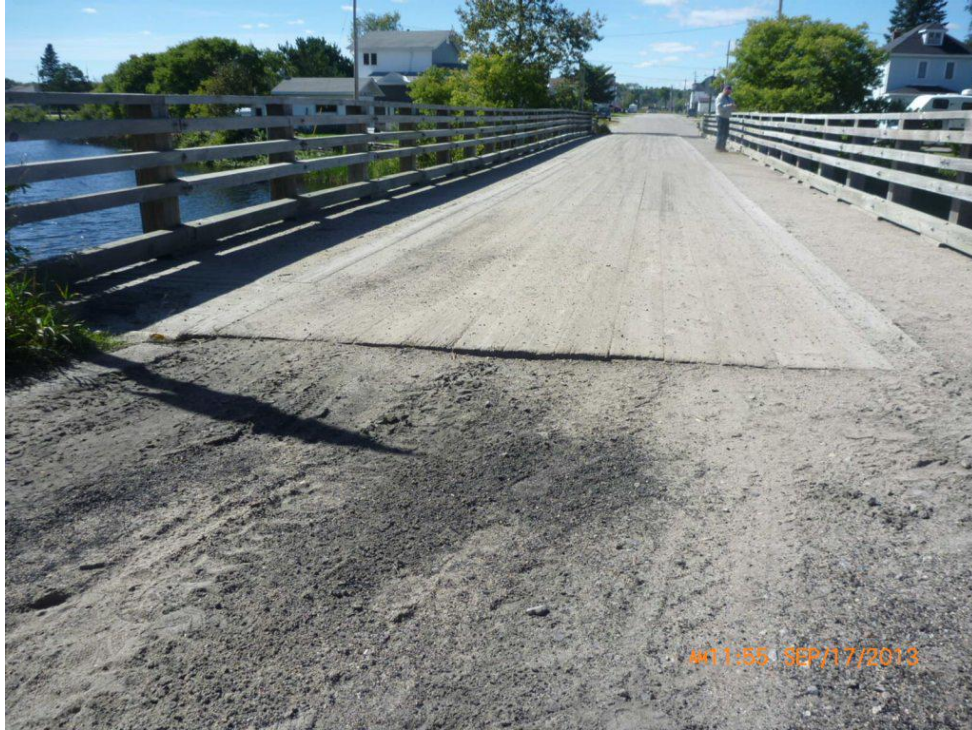
Comments: MISSING GRANULAR MATERIAL AT EAST APPROACH
