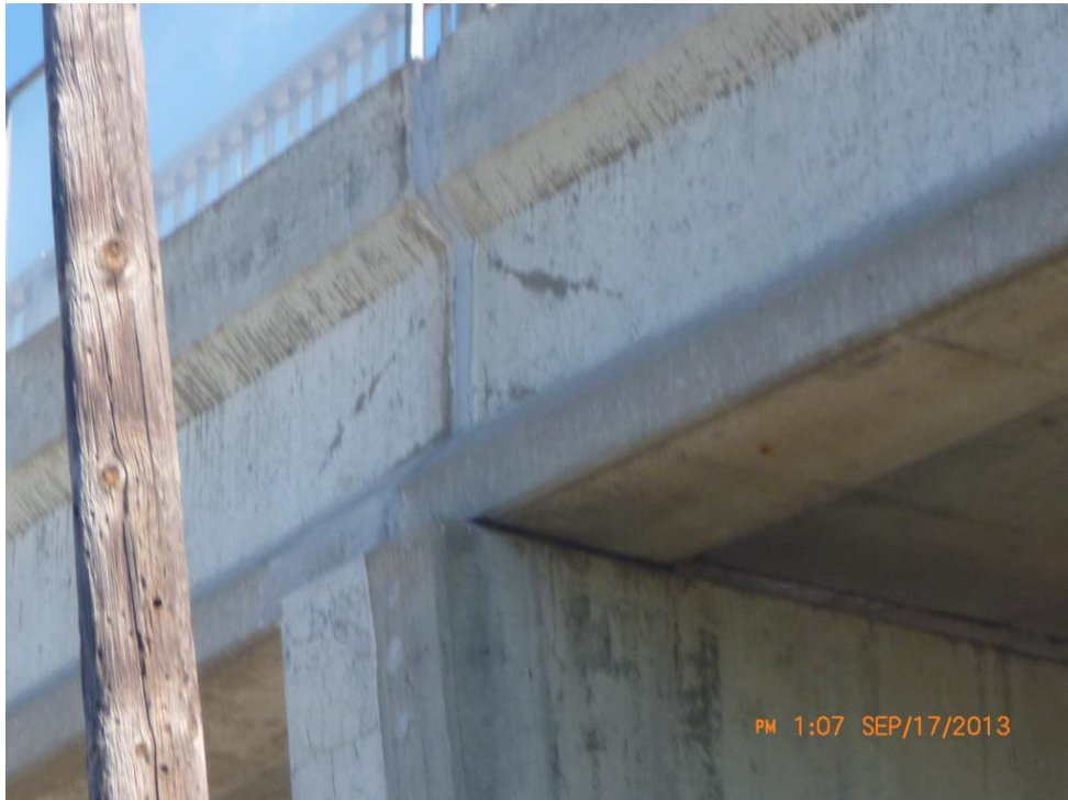
Comments: DIAGONAL CRACKING ON GIRDER END AT PIER
